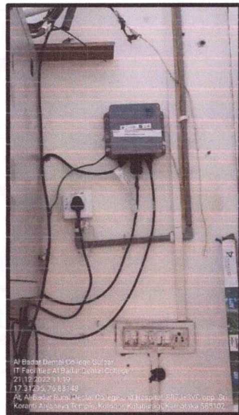
INSTALLED WIFI DEVICE
